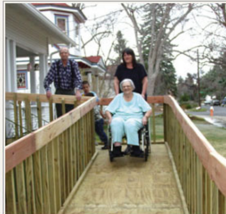
Volunteers from DaySpring Christian Church, Fort Collins, Colorado, have been building wheelchair ramps for area residents who are in need for several years.
